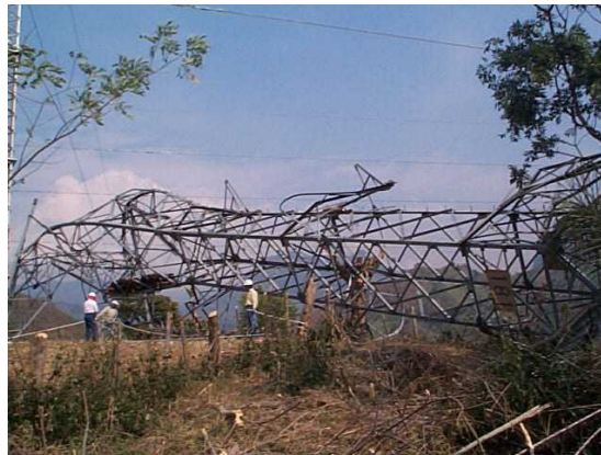
Fig. 1: Transmission tower destroyed by attack. Photo courtesy of ISA.
